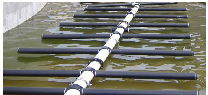
Fig. 1. Fine bubble air diffusion system consisting of a series of tube diffuser
