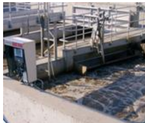
Figure 5. SC1000 controller on the tank by the strength installer
